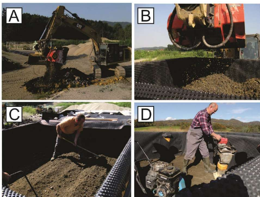
Figure s3 Different stages of a field preparation of geotechnical composites for the lysimeter experiments: Preparation of a composite, according to predetermined dry mass ratios and with addition of optimal amount of water, by the use of excavator mixing bucket (A), filling of the lysimeter with a layer of a composite (B), spreading of a composite in a layer of uniform thickness of 30 cm (C), and the final installation of the layer of a composite by a vibration compactor in box lysimeters (D).
