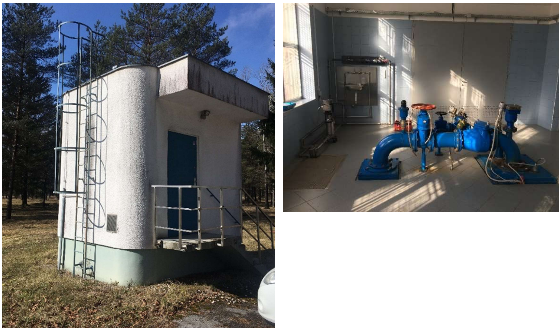
Figure 1.10: Wellfields Jarški prod and Šentvid in Ljubljana from outside and inside, respectively.
