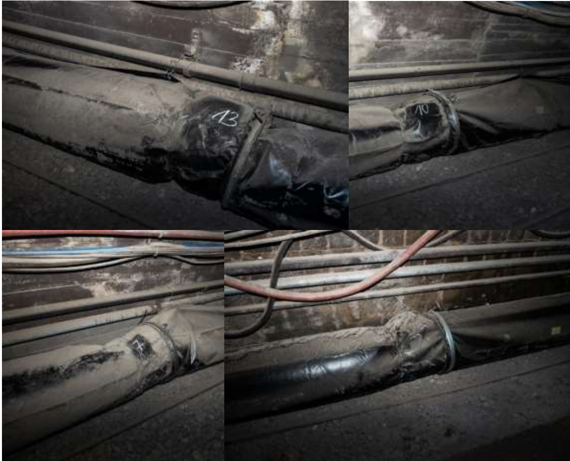
Figure 3.15: Constrictions before each joint of ducting between ducts.
