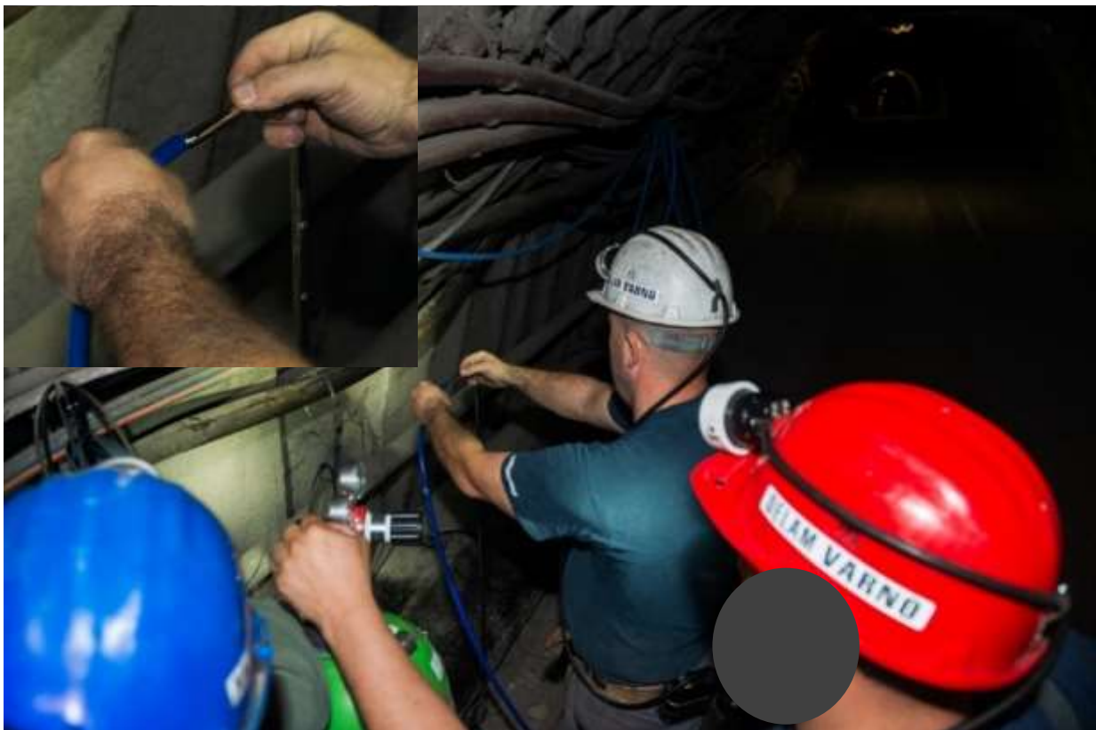
Figure 3.17: Adjusting the flow from the cylinder by carefully opening the pressure reducing valve with simultaneous measurements of flow velocity at the outlet by means of Pitot tube.
