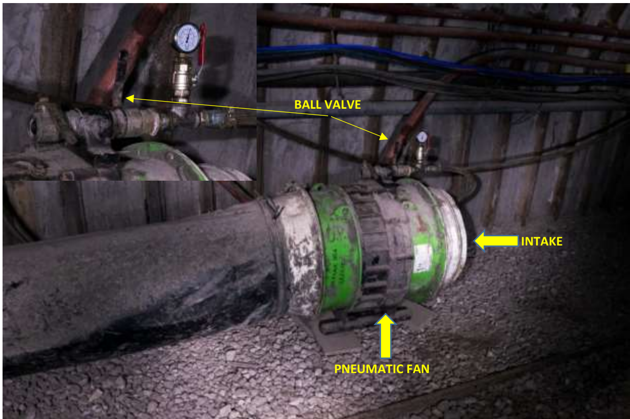
Figure 3.7: Pneumatic fan connected to the duct and ball valve for the regulation of fan power (drive with compressed air) and air flow.
