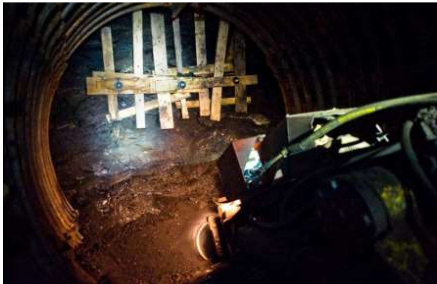
Figure 1.11: Development heading: cutting of the floor part of gateroad's profile with a roadheader GPK PV.
