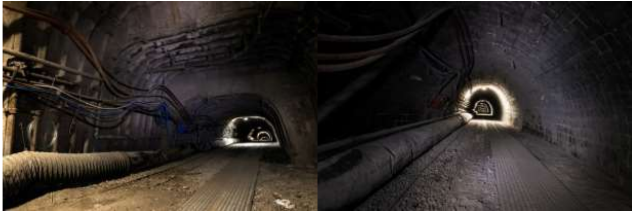
Figure 3.9: View of the ducting layout in the airway. Left figure: view of the ducting layout from monitoring location 1 in the direction of the end. Right figure: view of the ducting layout from the middle towards the end.
